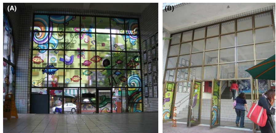
FIGURE 4 The un-openable glass wall at the front door of the ground floor of Building C, which obstructed the ventilation of underground floor classrooms. (A), before intervention and (B) after removal of upper two-third glass (replaced with insect screen)
