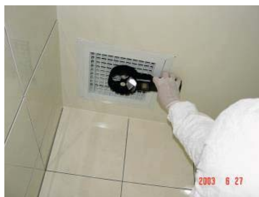
indirect measurement (rotary airflow meter)
